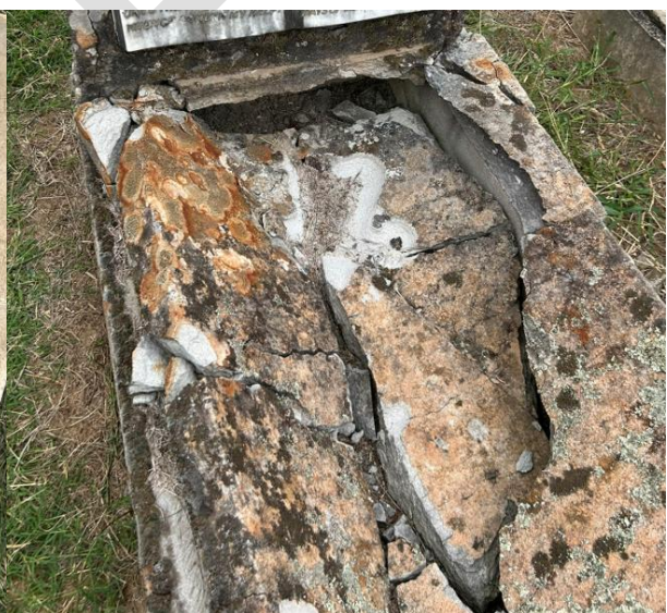
Figure 103: Example of a fractured stone ledger
