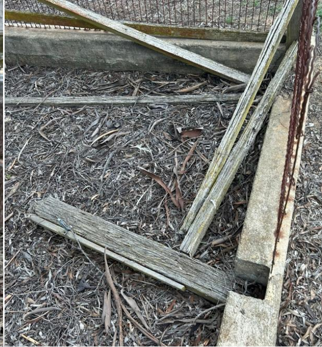
Figure 89: parts of a timber fence that has failed showing signs of biological growth and decay
