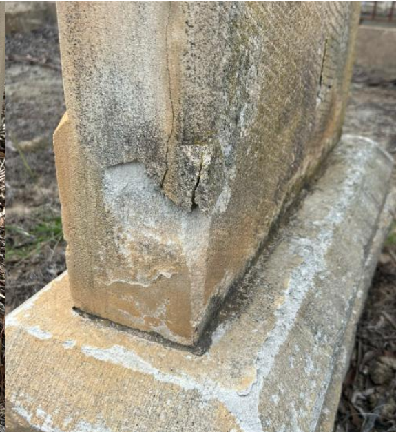
Figure 75: An example where blistering has resulted in parts of the stone becoming loose and breaking off
