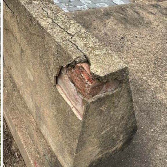
Figure 87: An example of a concrete render cracking and dislodging from the monument
