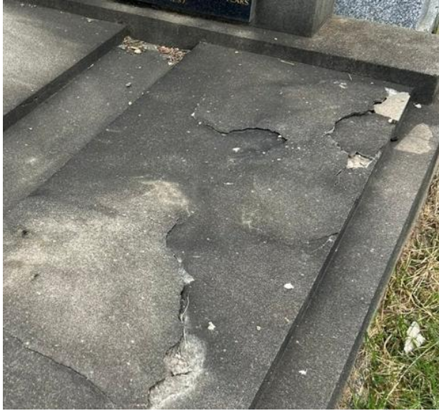
Figure 86: Cracking and discoloration of the concrete ledger
