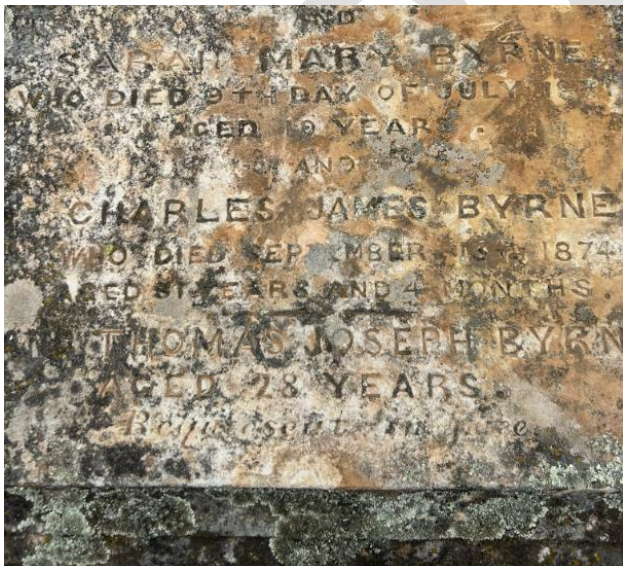
Figure 68: Discoloration of a sandstone element, the inscription remains legible on close inspection
