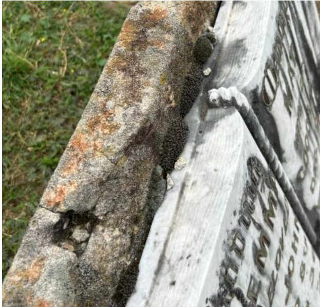
Figure 66: An example showing biological growths including lichen and moss causing discoloration of the sandstone
