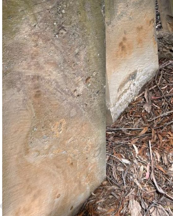
Figure 83: Examples of rising damp causing damage to the rear of sandstone monuments
