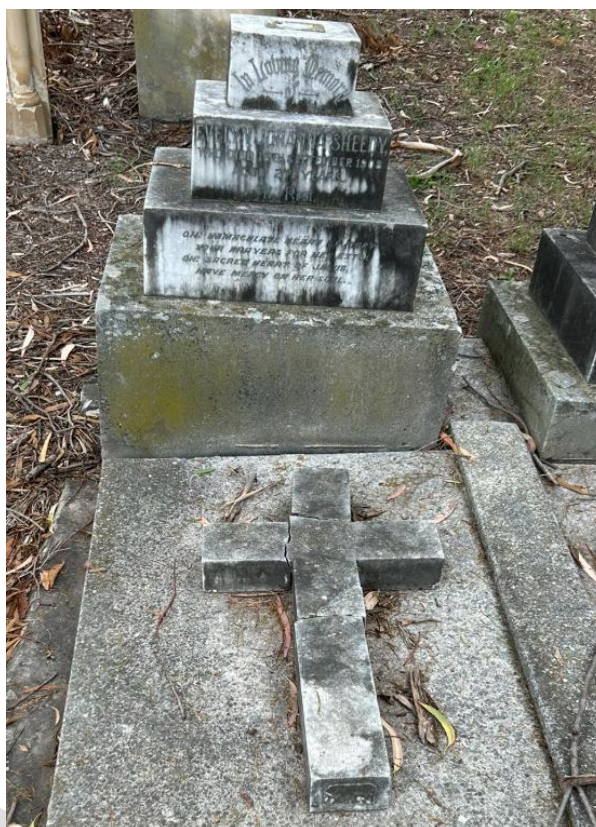
Figure 95: Example where a marble cross has come free from the monument and fractured but has been reassembled on the grave ledger
