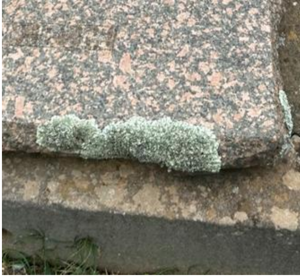
Figure 80: Example of a granite ledger displaying lichen growth
