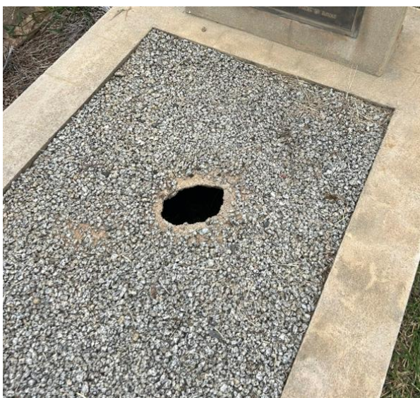
Figure 102: Example of a hole in a thin concrete and pebble floor
