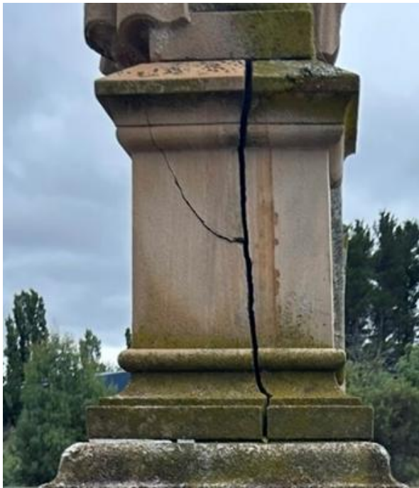
Figure 72: A sandstone element displaying a significant fracture
