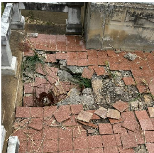
Figure 100: Example of a tiled floor where tiles are dislodged and the floor is damaged
