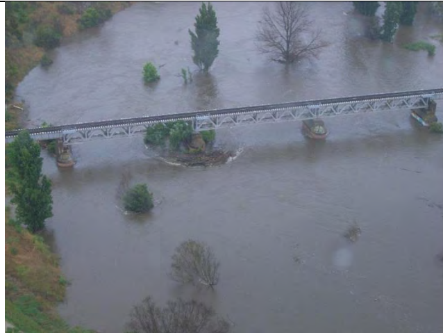
Plate B4.19 – 9/12/10 11:27 hours – Build-up of debris against Goulburn – Bombala Railway (Source: NSW SES)
