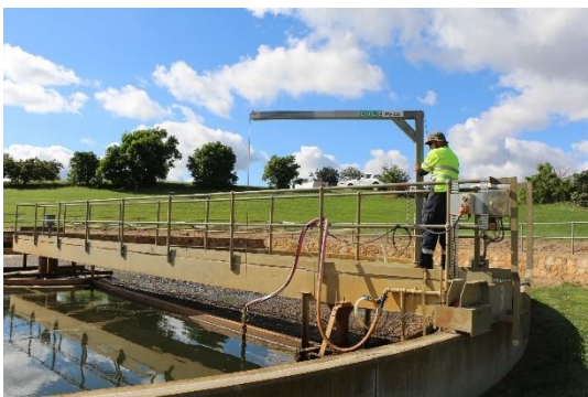
Queanbeyan Sewage Treatment Plant
