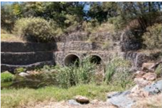
Stormwater drainage system
