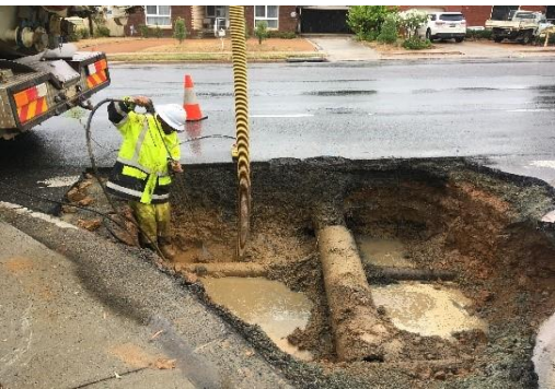
Cooma Street water main
